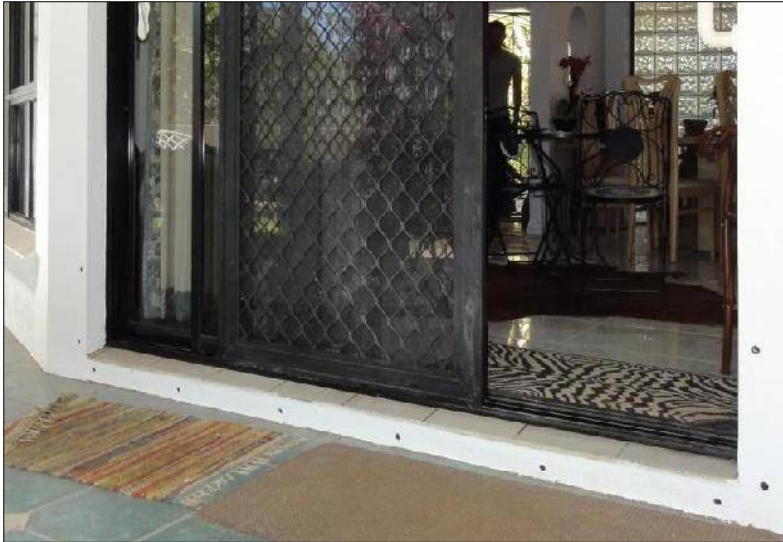
Figure 8: Drill holes around a resident's external doorway ready to install a sheet of marine plywood to help prevent water from entering the home
